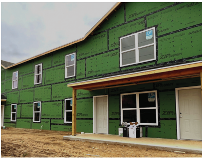
Two and a half months into the project and major progress is being made at 511 Division Street.
